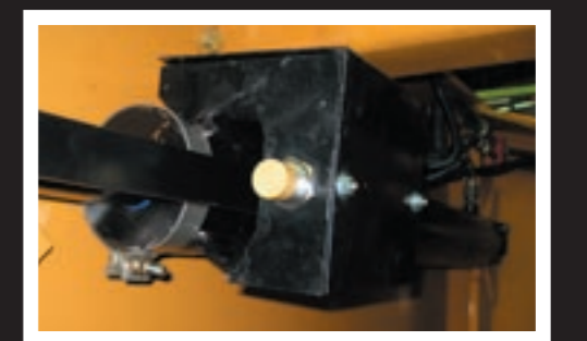
■ Self monitoring proximity switches monitor the movement of the ejector to keep operations in proper sequence
